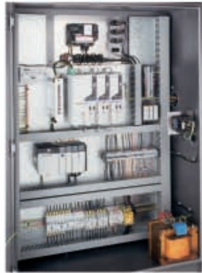
Interior view of Flowtronic 120 electrical cabinet
